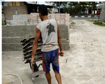
Figure 2 Workers transporting paving blocks ready for printing to drying places (see online version for colours)
