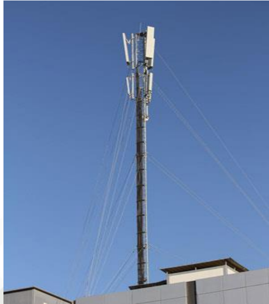
Gambar 2.10 Rooftop pole tower [13].
