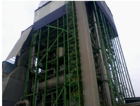
Gambar 4.2 Boiler PT. Indah Kiat Pulp And Paper Tbk Perawang Mill.
