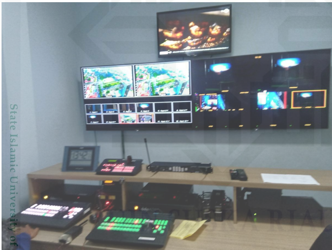
Gambar 3. Ruang dan Alat Master Control Room (MCR)
