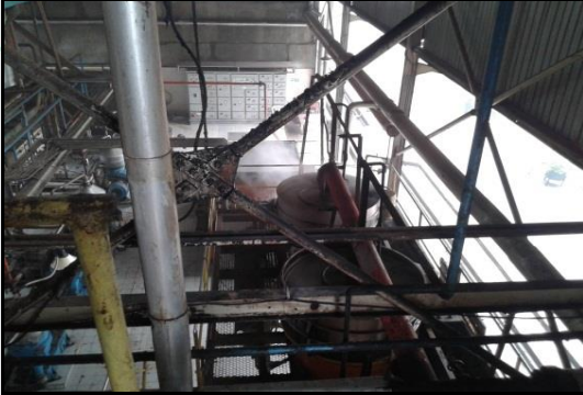
Sand Trap Oil Tank
