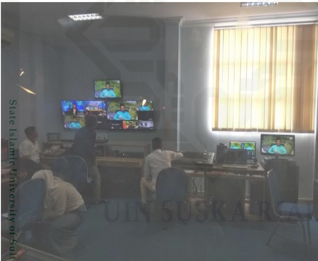
Gambar 10 : Master Control Room (MCR)
