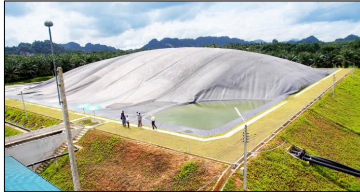
Gambar 2.5 Digester Covered Lagoon [3].
