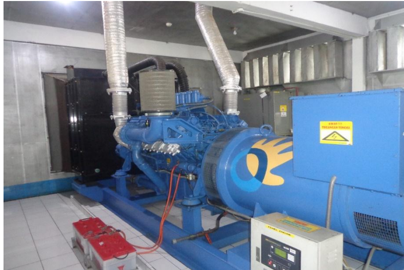
Gambar 2.3 Genset Leroy Somme / LS656-C6/4
