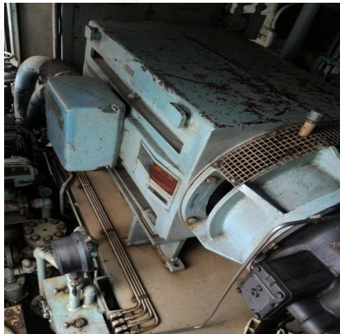
Gambar 2.21 Motor Starting PLTG PT. Riau Power Sumber : PT. Riau Power Pekanbaru (2016)
