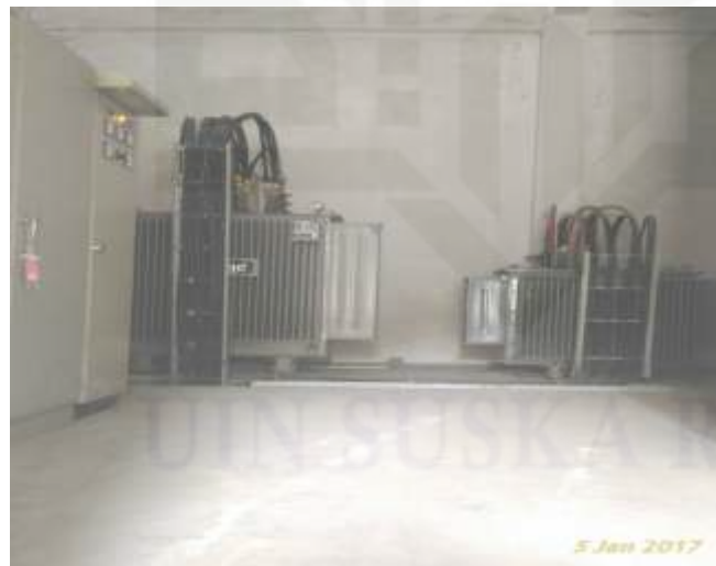
Gambar 2-12 Transformator distribusi 20 kV UIN Suska Riau.
