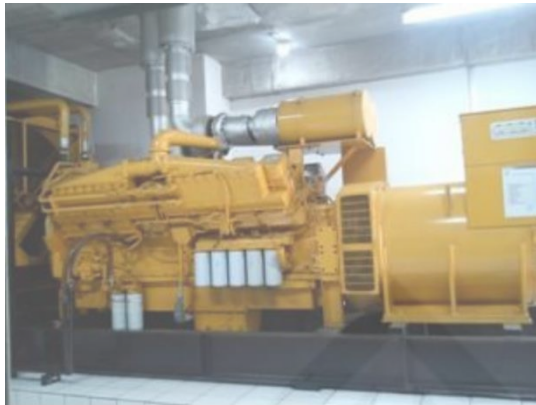
Gambar 2.2 Genset (Generator Set)
