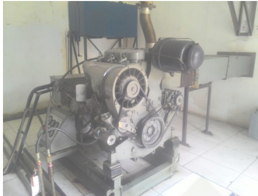
Gambar 2.4. Genset Deutz model OJDS 25 SB (Sumber gambar: PT. Telkom Arnet Ridar)
