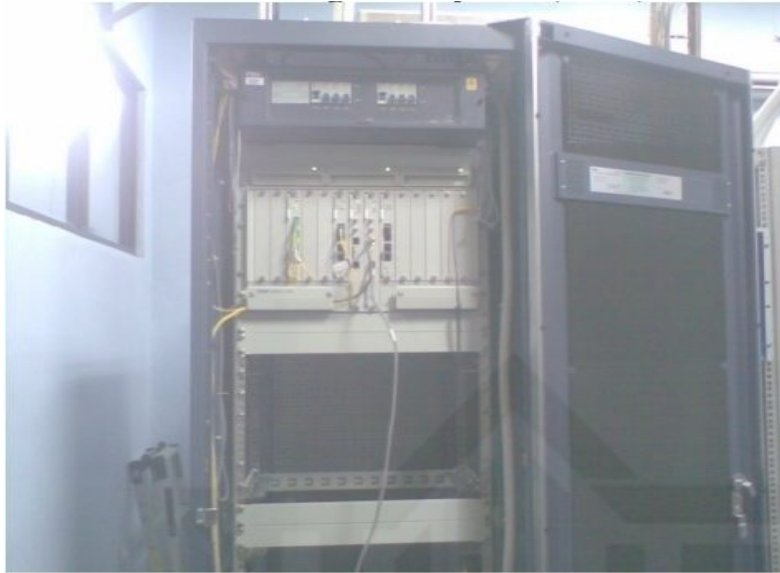
Gambar 2.8 Optical Line Terminal (OLT)
